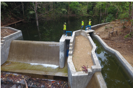
A micro-hydro power plant being built in Lubuk Bangkar Village, Jambi for communities (Photo: UNDP)
